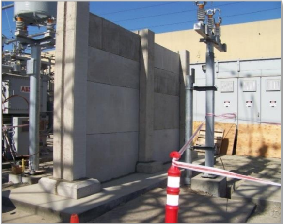
Physical Firewall at Electrical Substation
